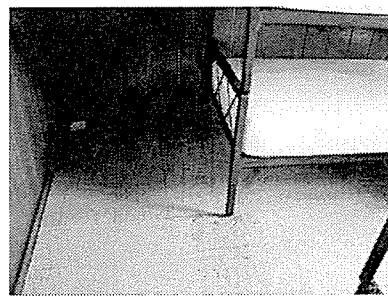
Photo #52 Bedroom. Asbestos containing black mastic under the 12"x12" cream colored tile.
