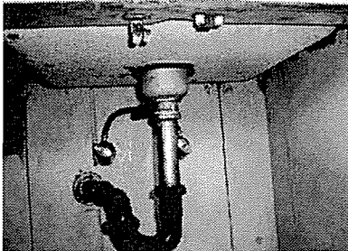
Photo #60 Asbestos containing gray undercoating sink mastic.
