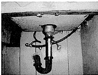
Photo #48 Asbestos containing gray undercoating sink mastic.
