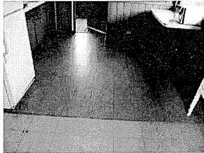
Photo #9 Kitchen. Asbestos containing tile and mastic under the 12"x12" brown speckled tile.
