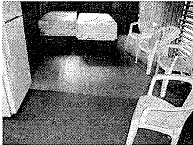
Photo #45 Bedroom by the kitchen. Asbestos containing tile and mastic under the 12'X12' cream tile with tan specks.
