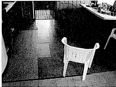
Photo #21 Kitchen. Asbestos containing tile and mastic under the 12"x12" brown speckled tile.
