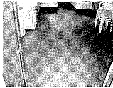
Photo #58 Asbestos containing black mastic under the 12"x12" cream colored tile with tan specks.
