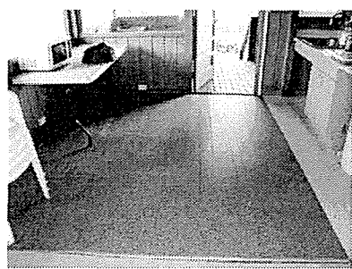
Photo #16 Kitchen. Asbestos containing tile and mastic under the 12"X12" brown speckled tile.
