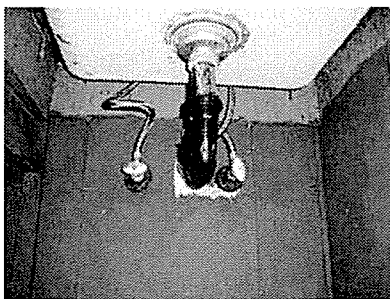
Photo #6 Asbestos containing gray undercoating sink mastic.
