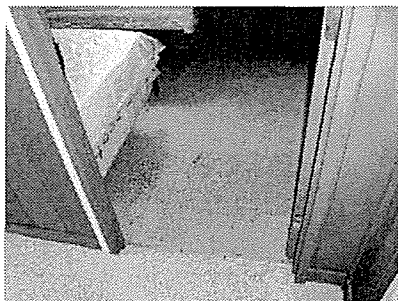
Photo #15 Bedroom. Asbestos containing 12"X12" light-gray tile with white specks.
