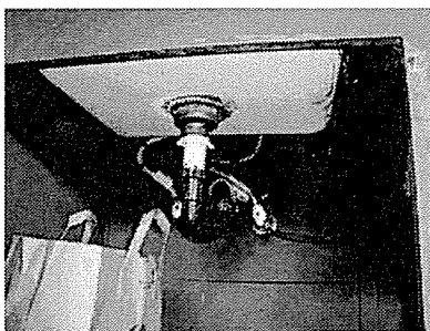
Photo #36 Asbestos containing gray undercoating sink mastic.
