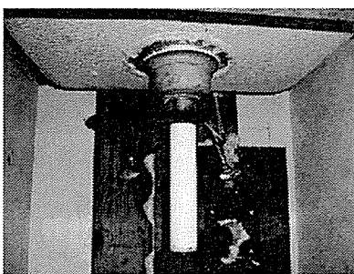
Photo #42 Asbestos containing gray undercoating sink mastic.
