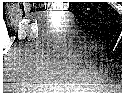
Photo #34 Kitchen, Asbestos containing tile and mastic under the 12"x12" brown speckled tile.
