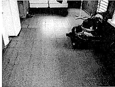
Photo #27 Kitchen. Asbestos containing tile and mastic under the 12"x12" brown speckled tile.
