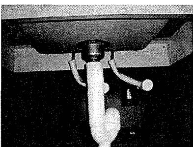
Photo #18 Asbestos containing gray undercoating sink mastic.
