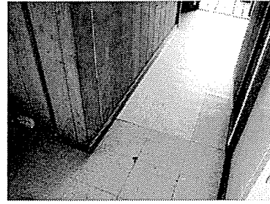
Photo #10 Hallway. Asbestos containing 12"x12" light-gray tile and brown mastic.
